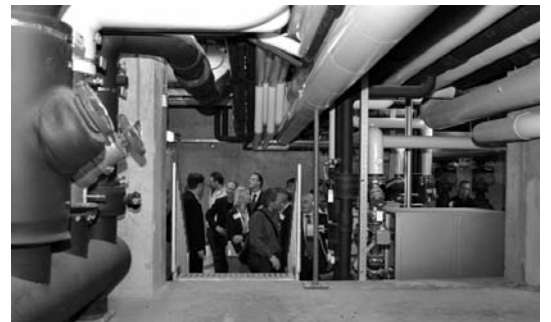
Figure 9: Facilities of the Minewater Project at the Gen Coel Energy Center in Heerlen, where a technical tour was offered during the Conference.
